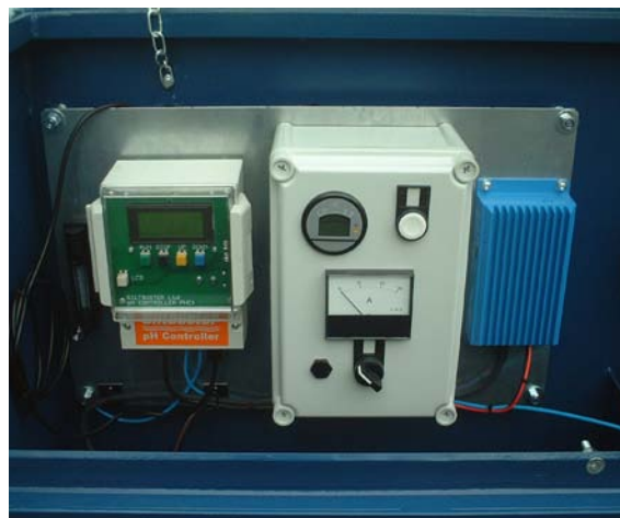
pH Controller, Battery Charger and Control System ▲
